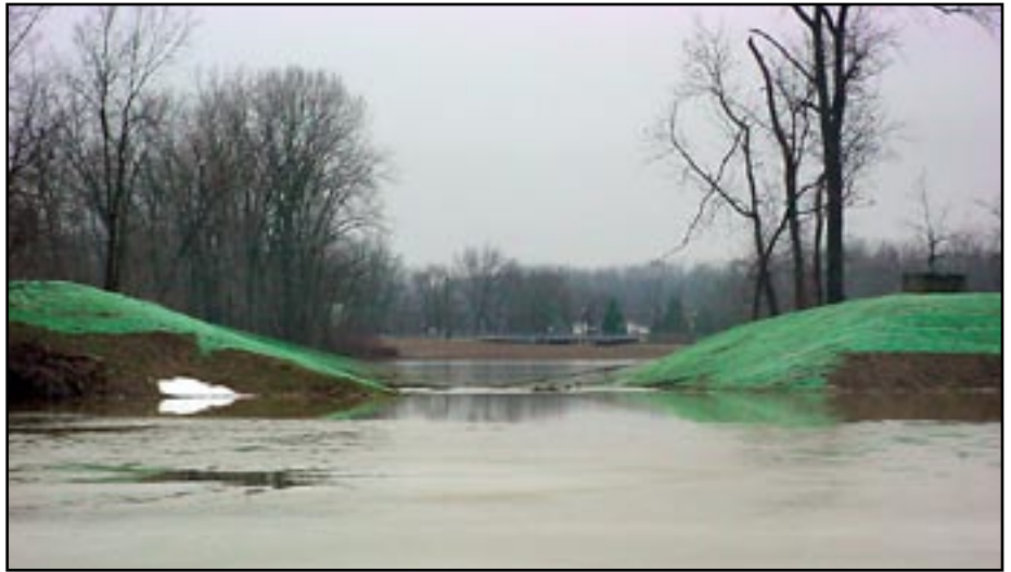
Breach in embankment at Leighty Lake near Newport.
